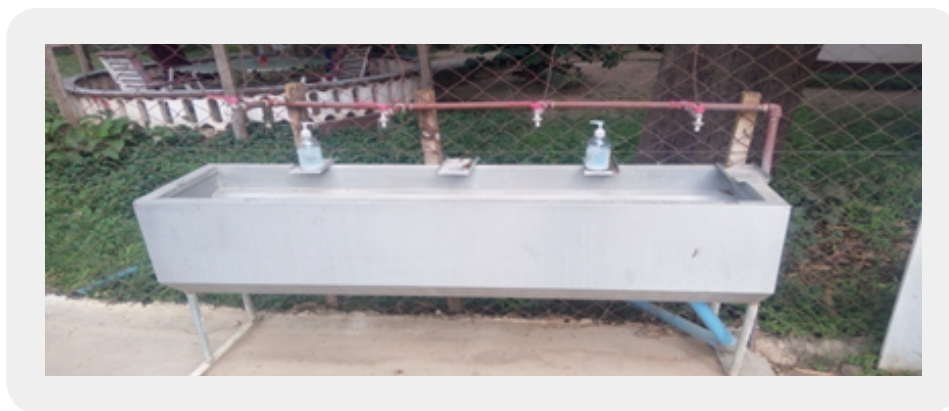
Figure 2: Handwashing facility at the main gate of SFRH.
